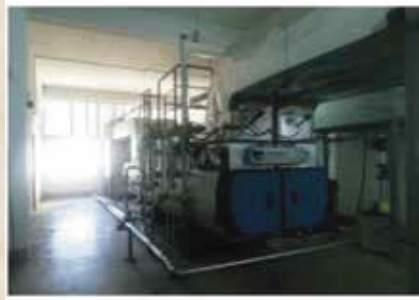
Exhausted Gas Boiler (Reduce 3.00%)
